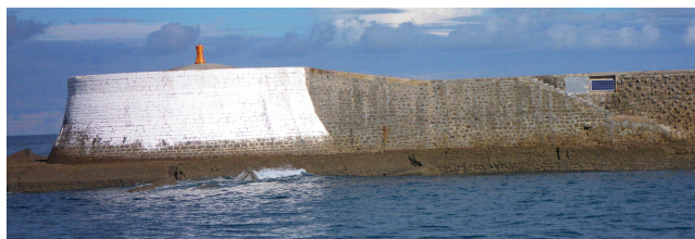
FIGURE 3. The dyke (view of the protected side) with electrical instrumentation setup on the right.
